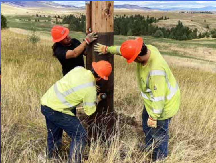
Micheal Fisher, Kaden Blixt and Tristan Garcia Installing Fire Mesh. Photo by Leon Wieder
